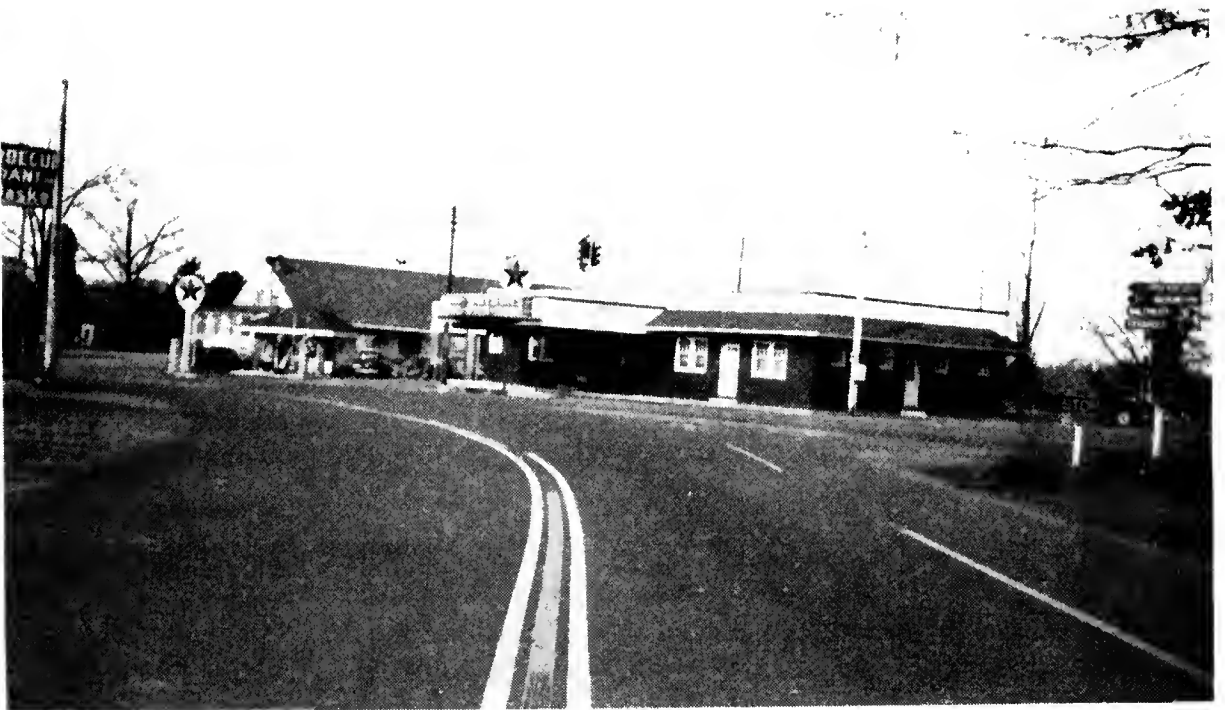
WIDENING AND RESURFACING INTERSECTION OF MD. ROUTE 4 AND MD. ROUTE 416, AT WAYSON'S CORNER
